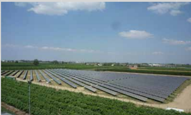
Free-field installation, Italy
